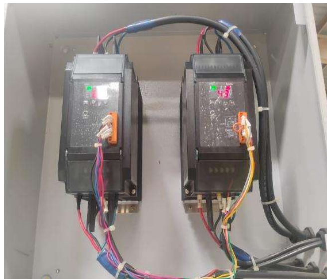
Thyristor control, Chennai
