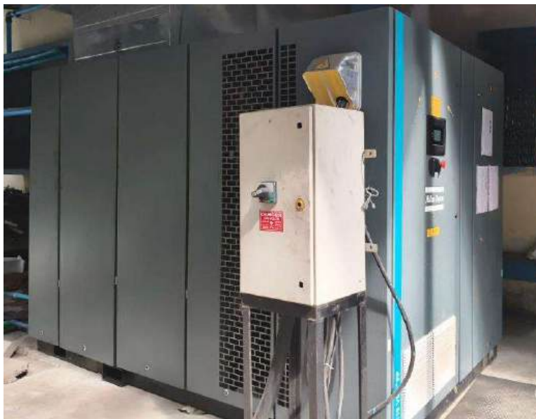
New Compressor at Madurai Plant
