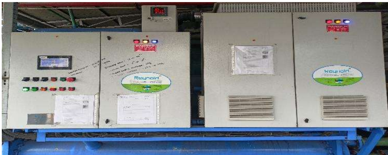
Chiller at Madurai Plant
