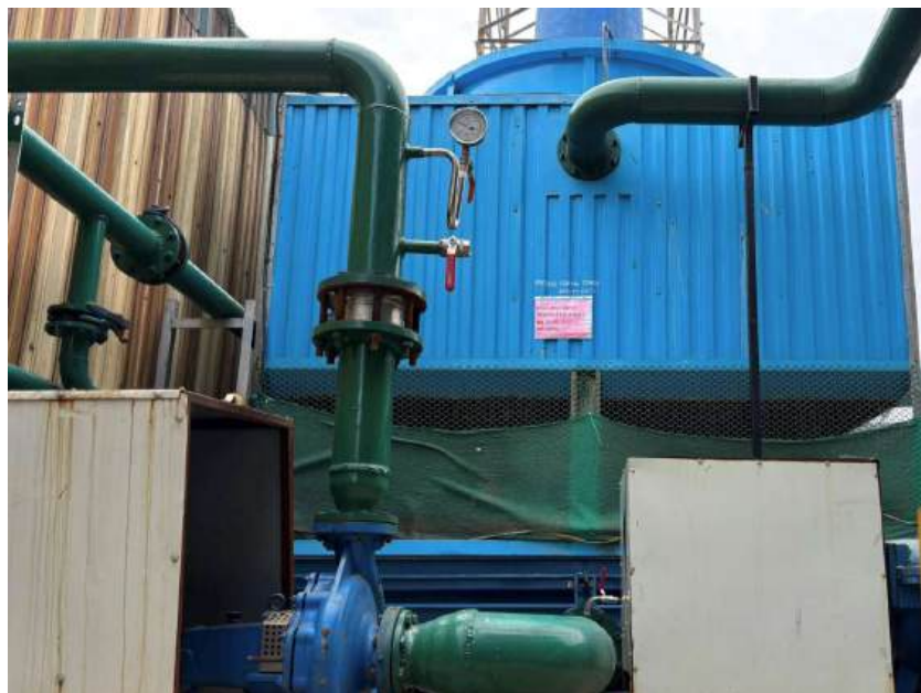
Cooling Tower at Madurai Plant
